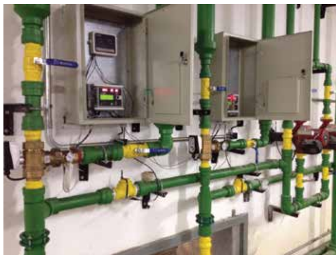
Installation at Rio de Janeiro hotel
